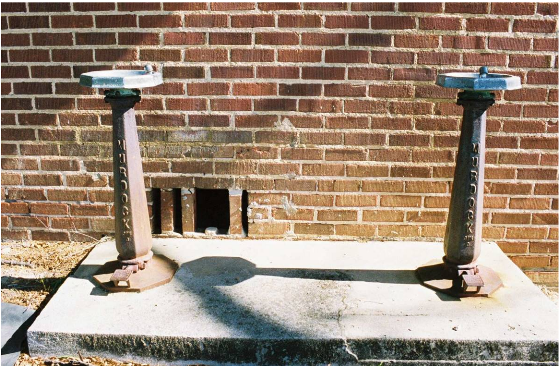
Plate 204. Spring Hope School: early or original Murdock fountains behind south rear of school
